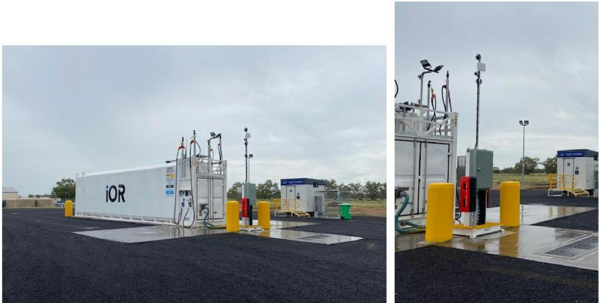
Figure 3: Example lighting around tank (source: IOR)
