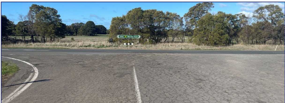
Figure 12: Hopkins Falls Road/Princes Highway Pavement Condition
