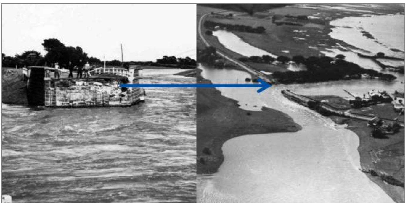
Figure 7. The Rosebrook Bridge along the Princes Highway washed away in the 1946 flood.
