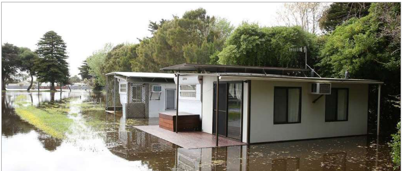
Figure 16. A cabin impacted by flooding at the Port Fairy Gardens Caravan Park during the October 2020 event.
