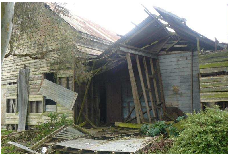
butter factory collapsed section, 2012
