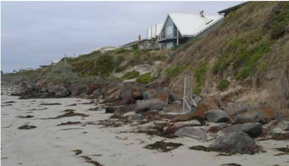
Figure 4-2 Northern End of Seawall of Sub-Standard Construction
