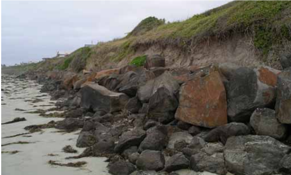
Figure 4-1 Section of Seawall of Sub-Standard Construction
