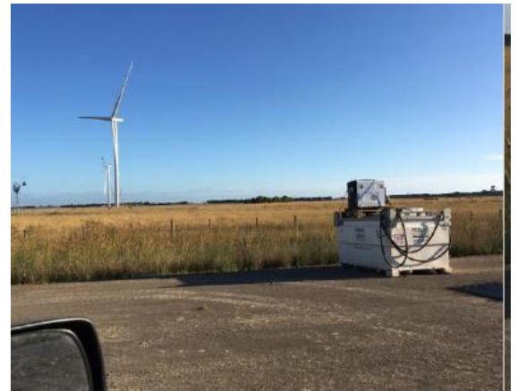
Acciona's diesel fuel bowser set up on a road in Kolora, to service the Mortlake wind farm construction works during the fire danger months of Jan-Feb 2021.
